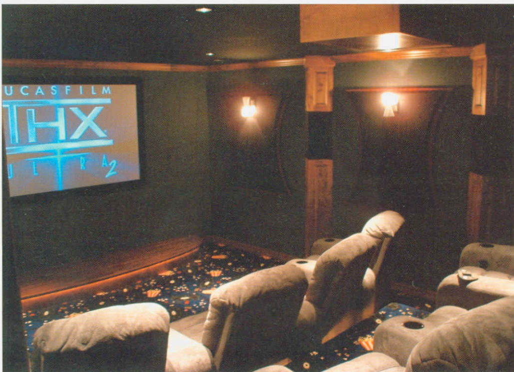
Escaping into the world of cinematic art is easily achieved in this private state-of-the-art cinema room designed and installed by CinemaQuest, Inc.
